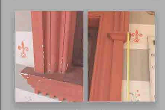
The redesign of the door and window frames of the porch highlighted the different size and decoration of the frames.
