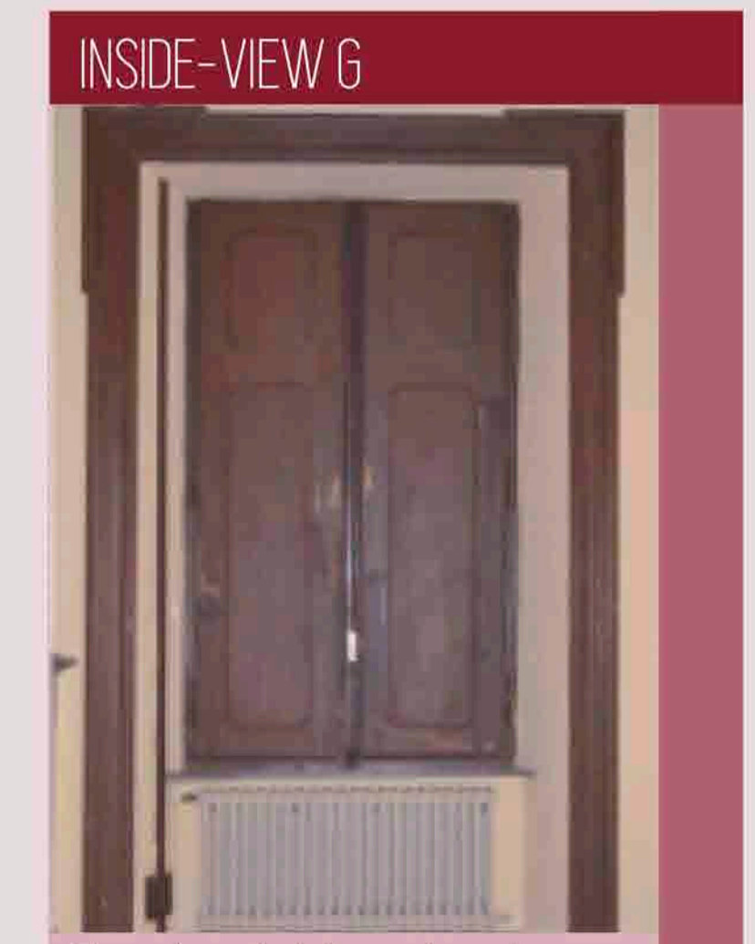
The wall on which the window is located is the least thick of the two halls: this portion is in fact the last one built during the castle's revolution phase.
